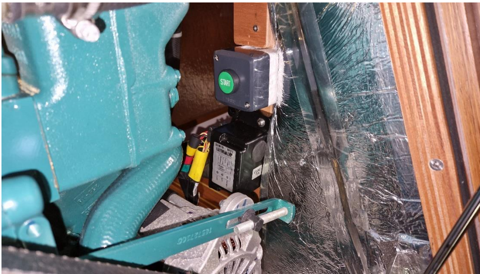
Emergency START button
